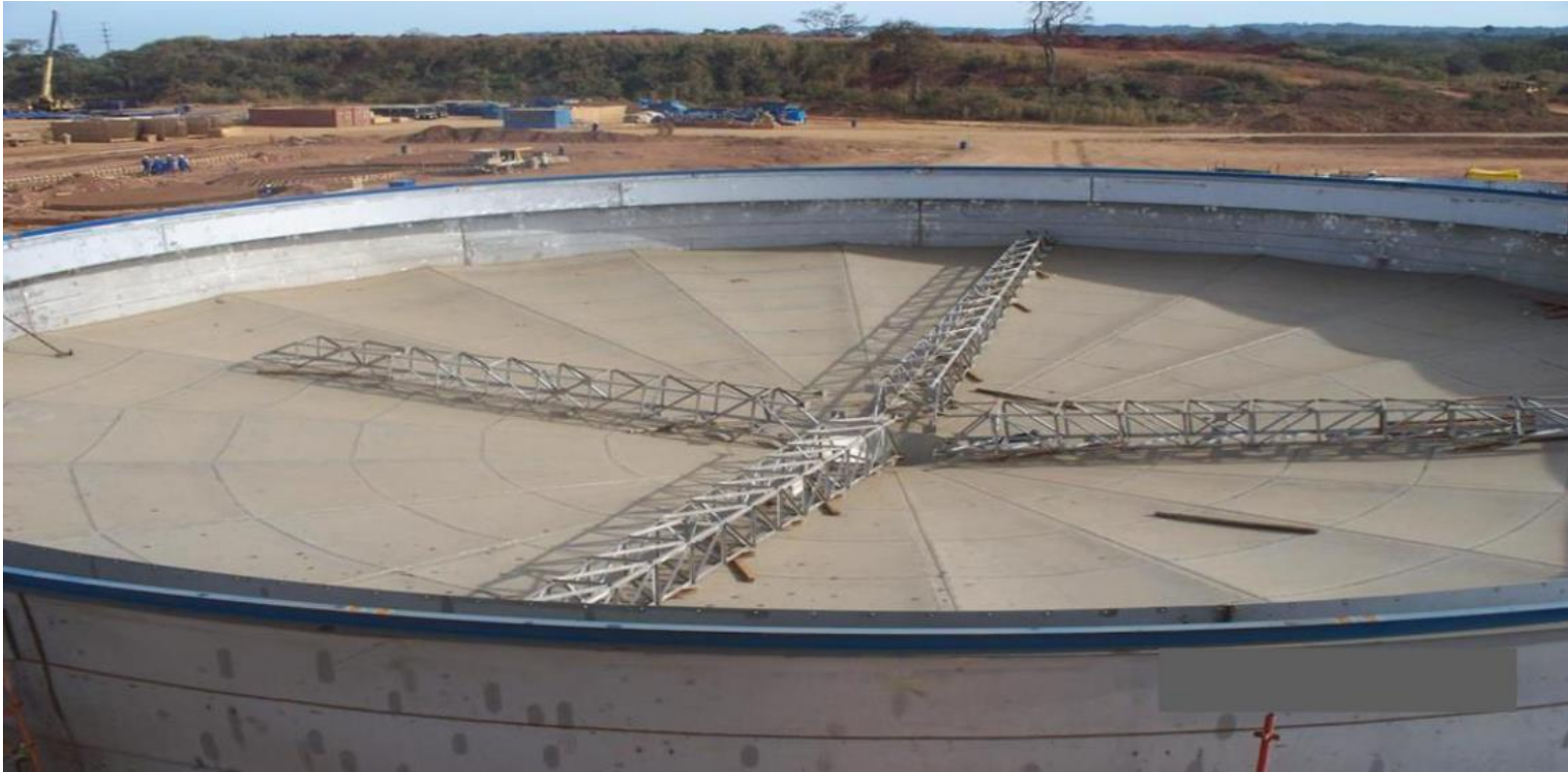
Counter Current Decantation (CCD) tank in mining industry
