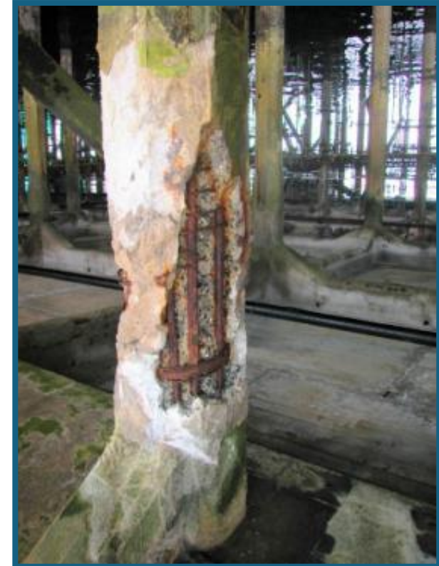
Chloride induced corrosion in a coastal environment
